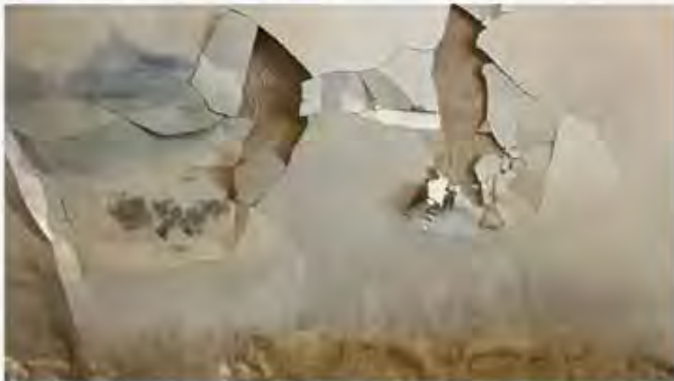
Mohammed's bedroom wall in Luton is covered in damp and mould as a result of botched insulation
