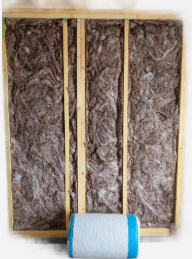
Plot X – insulation continuity observed.
