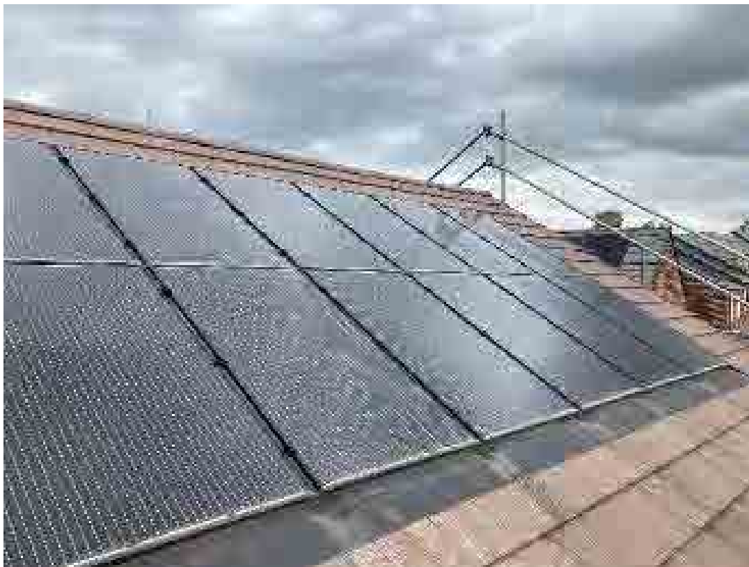
Solar panels to rear
