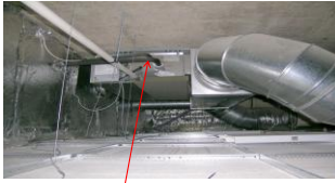
Refrigerant pipework ( not water)
